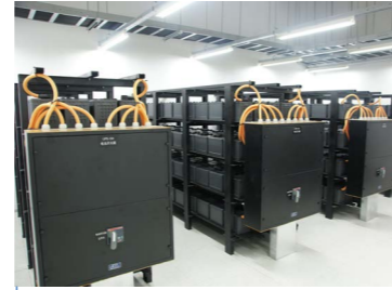
UPS Battery System
