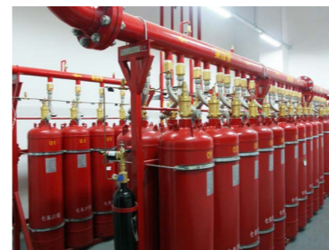
Gas Suppression System
