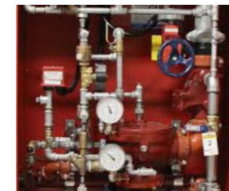
Pre-action Sprinkler System
