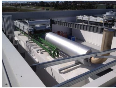
Canberra Data Centre, Australia
